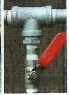
Galvanized Steel & valve
